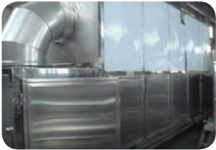
冷冻压缩机组 Refrigeration device
